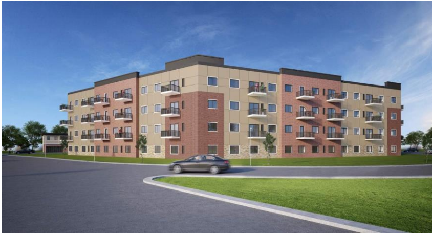
"The River" Apartments, under construction on the former south mall parking lot
